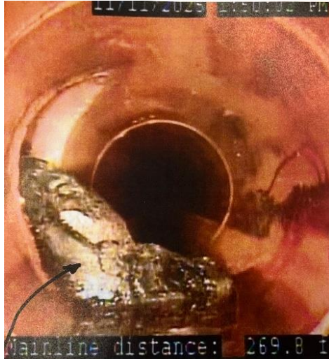
Sewer debris exiting from private residence
